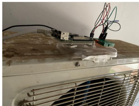
Figure 5. Location of the solution on the air conditioner
