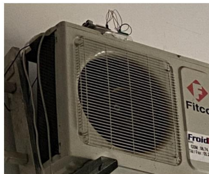
Figure 9. Location of the box during monitoring
